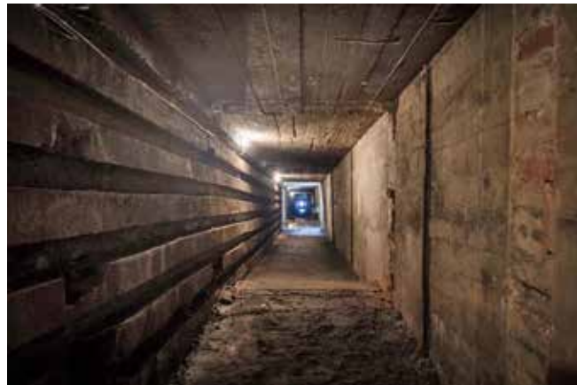
The cable tunnel at the Fly Trap that leads to the valley below and its coal mines. Cable trays on the left-hand wall. Photo Mike Scott
